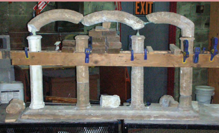
⤎ Recasting, filling and repairs were made to the heavily damaged Webb family monument during the winter and spring of 2009.
