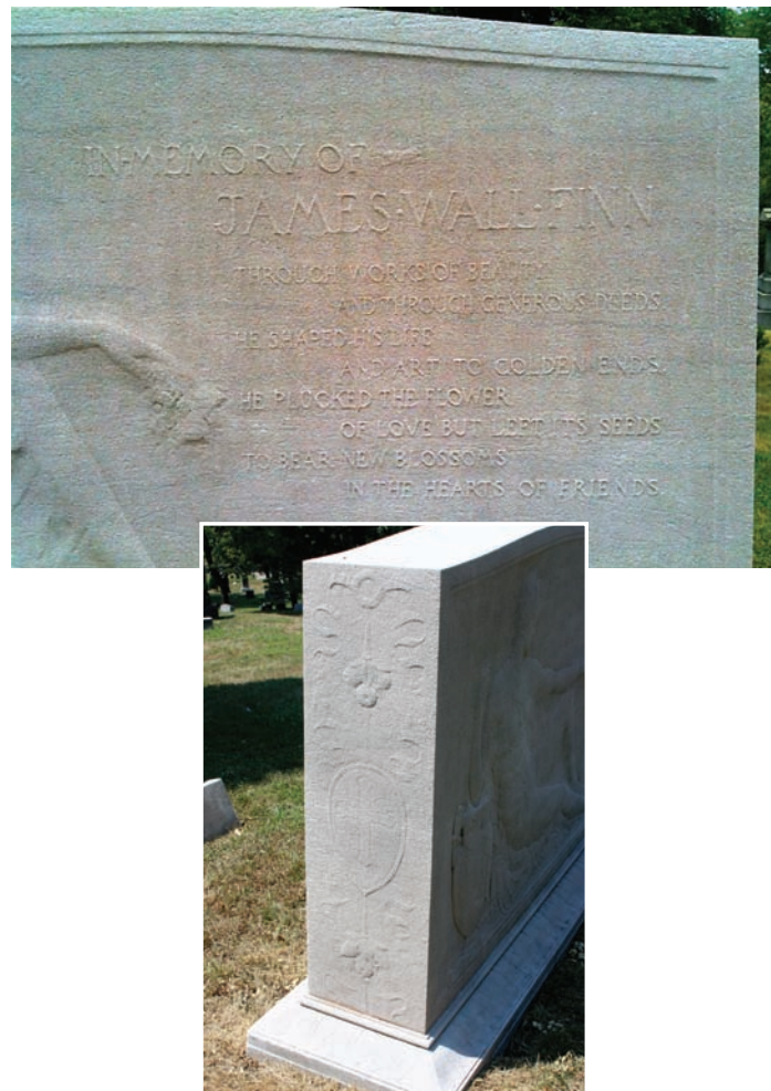
[Opposite page] The monument to James Wall Finn by fellow artist Frederick MacMonnies before and after cleaning.
