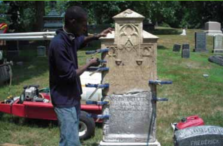
^ [above and below] Omri Faroul, working on the grounds, v repairs damaged headstones and monuments.
