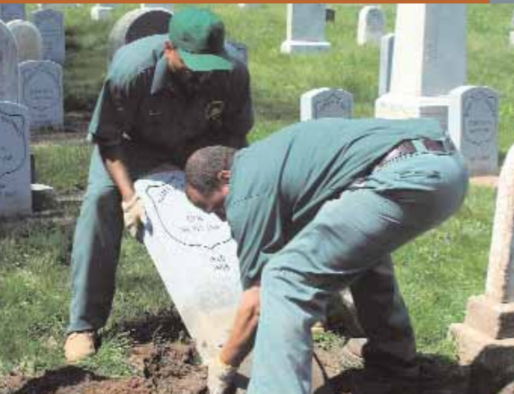
≈ Elvis Merizalde and Felipe Hernandez installing a gravestone in the Civil War Soldiers’ Lot.
